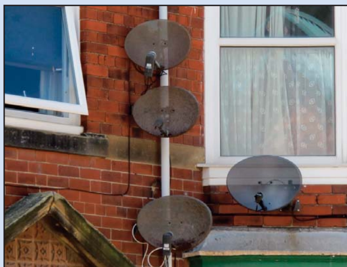
Untidy impact of multiple satellite dishes
