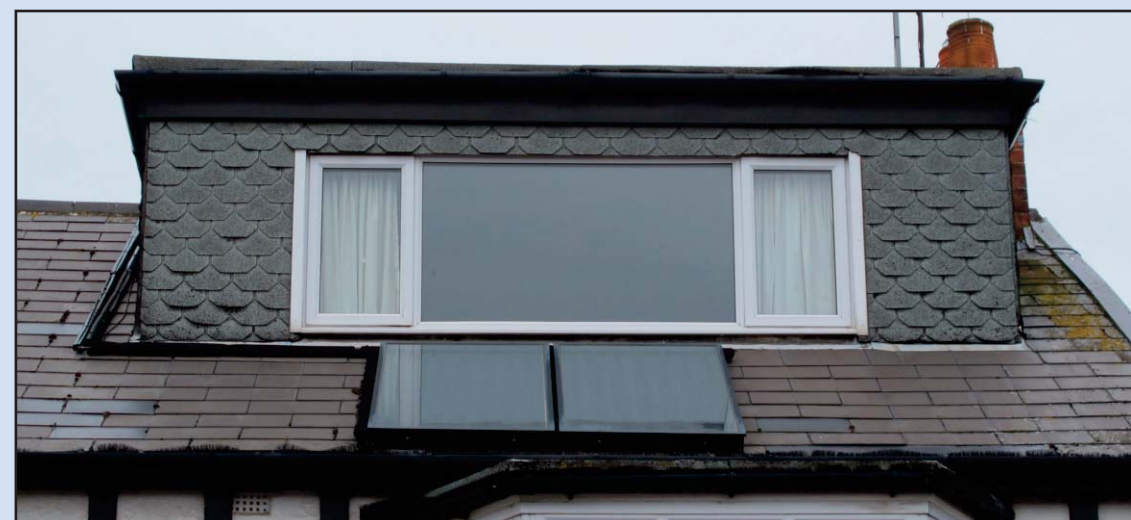
Overbearing and unsympathetic dormer window
