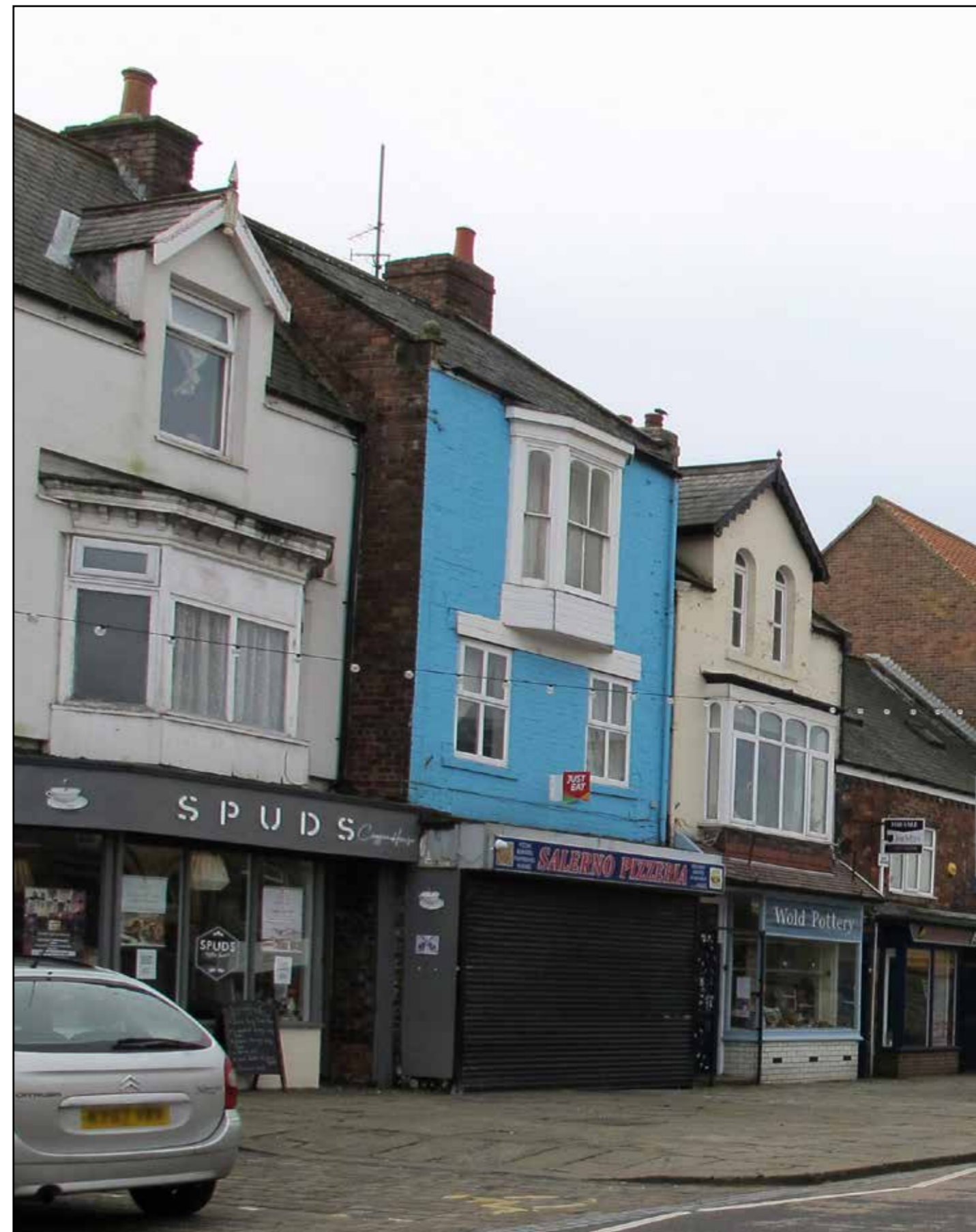
Obscured Facing Materials, Loftus Market Place
