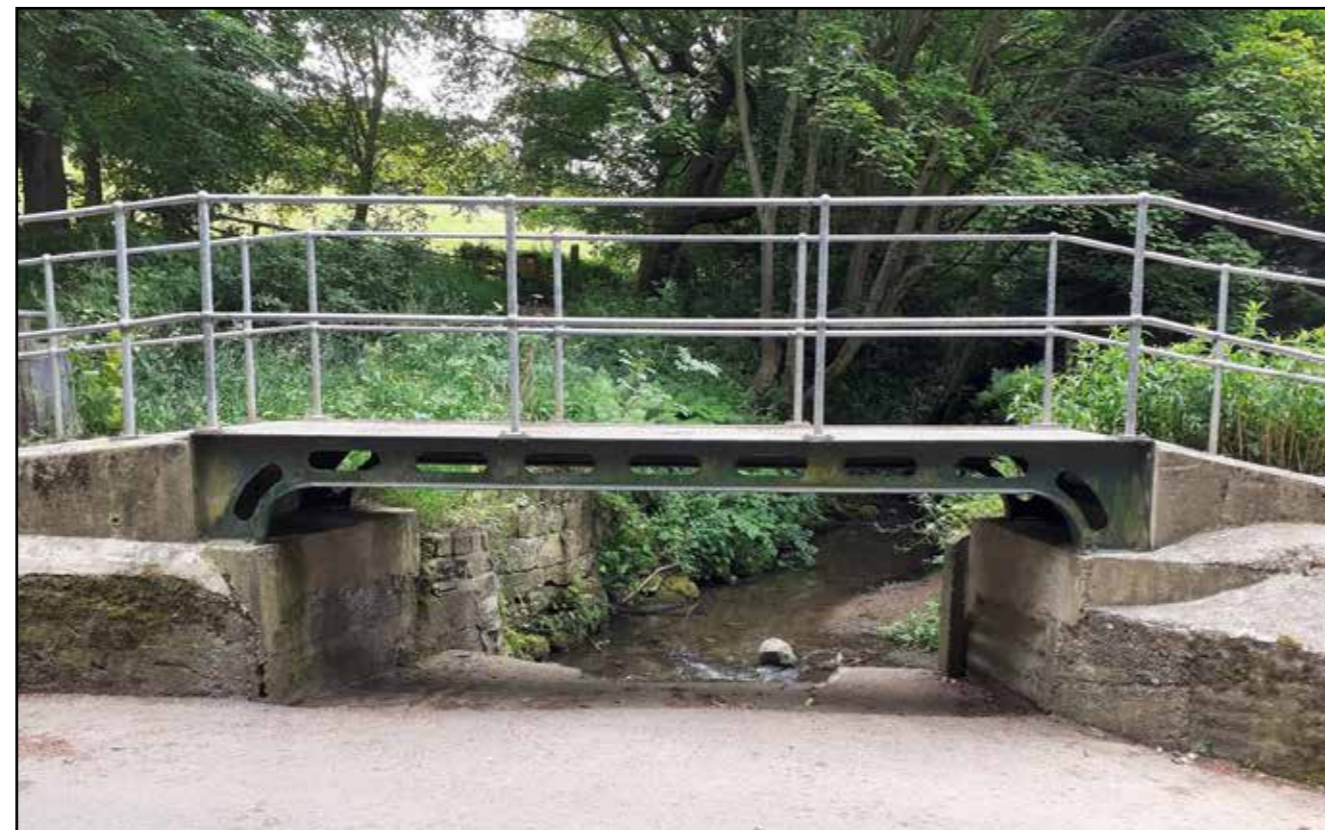
Unsympathetic steel bridge and railings, Dam Street
