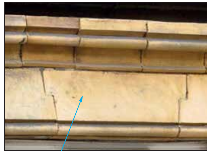
Stone used for bands and dressings around windows and doorways and frequently for bay windows.
