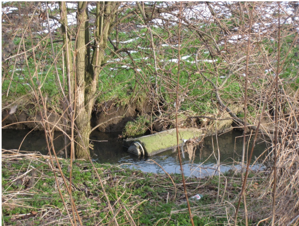
Figure 14 - Surface water sewer entering Chapel Beck
