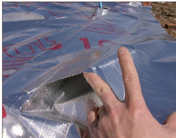
Figure A4.78 Gap in jointing over wall cavity big enough to insert fist (courtesy Smith Grant)
