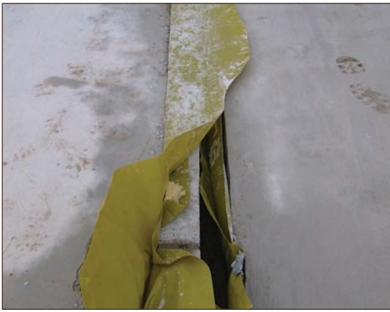
Figure A4.79 Gas membrane not continuous over internal wall. It had been deliberately cut open for unknown purpose (courtesy Smith Grant)
