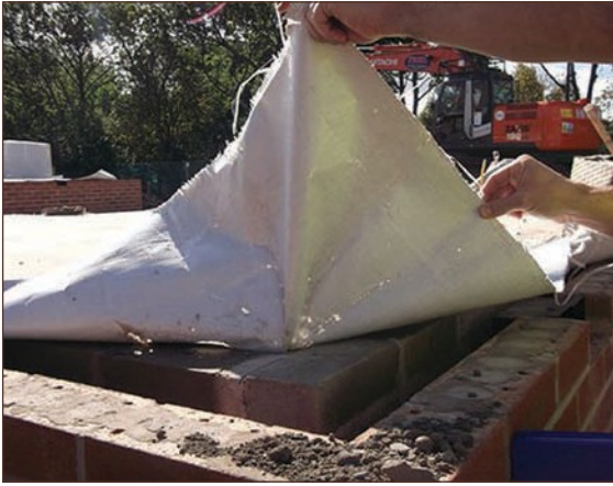
Figure A4.49 Lifted gas membrane at corner position. Light penetrating through confirms damage to aluminium internal core layer (courtesy NHBC)
