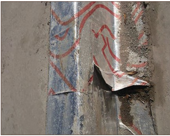
Figure A4.55 Gas membrane at stepped junction of slab to integral garage, appears to be susceptible to tearing when screed is poured. Screed may also weigh down on gas membrane if fitted too tight (courtesy NHBC)
