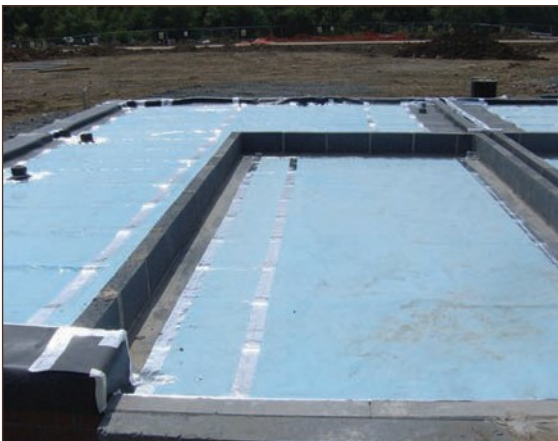
Figure A4.11 Gas membrane continued through cavity wall and above air bricks (courtesy Hydrock)
