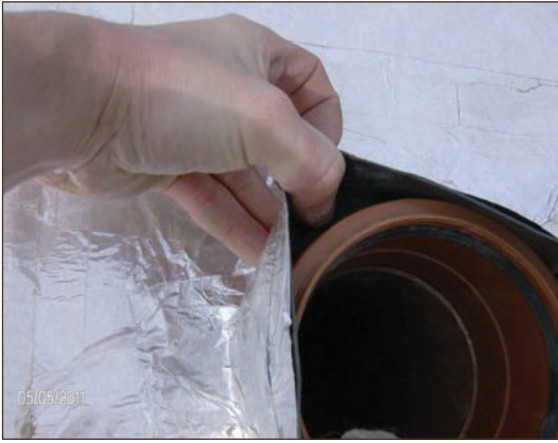
Figure A4.73 No bead of double sided butyl tape provided between interfaces of ID top hat and OD service pipe: cannot be compressed enough to form seal (courtesy Smith Grant)
