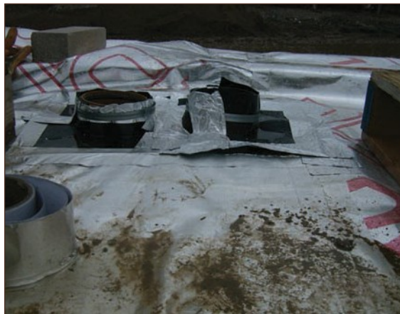
Figure A4.72 Joint between top hat and gas membrane has lifted due to poor fit and attempt to construct in very wet conditions (courtesy Smith Grant)
