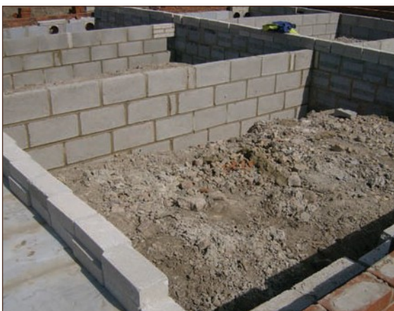
Figure A4.89 No ventilation in internal sleeper wall (courtesy Smith Grant)
