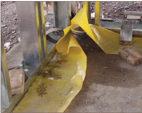
Figure A4.81 No seal to perimeter pipe (courtesy PAGEotechnical Ltd)
