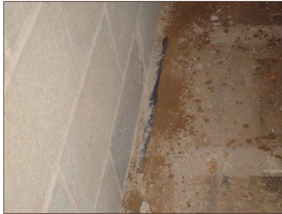
Figure A4.64 Insufficient length of gas membrane protruding through wall to overlap with gas membrane within building (courtesy Card Geotechnics Limited)
