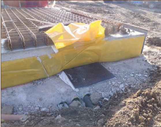
Figure A4.7 Geovent protruding out of the frontage of the unit. Gas membrane along the sides of the slab preventing lateral gas ingress (courtesy Alderburgh Group)
