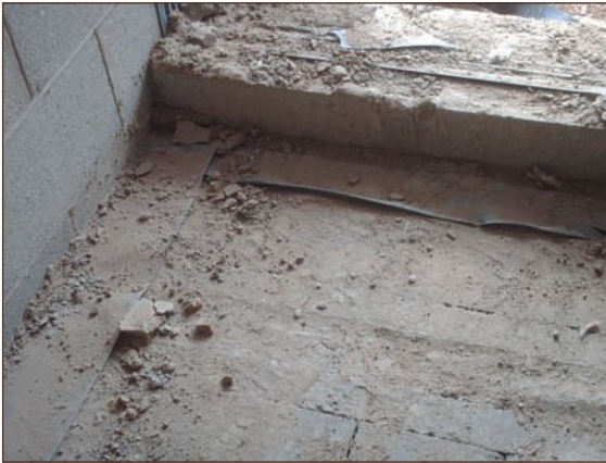
Figure A4.63 Absence of surface preparation prior to laying of gas membrane, debris likely to pierce gas membrane (courtesy Card Geotechnics Limited)
