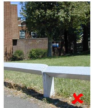
Fig 128. A repair using wrongly dimensioned timber.
