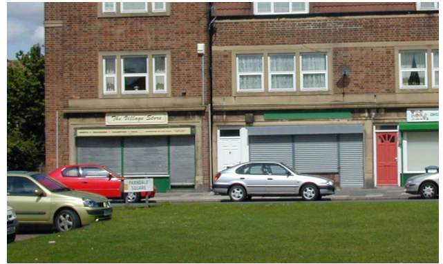
Fig 62. Solid shutters harm the streetscape and can give concealment to break-ins at rear. Internal grille-shutters avoid this.
