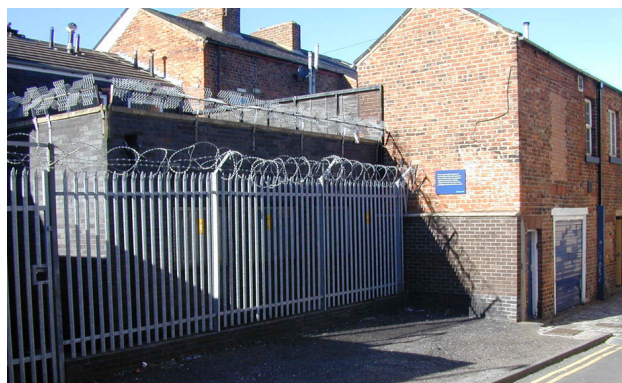
Fig 57. The gross negative impact of crude security. Thought at the design stage removes the need for such desperate measures.
