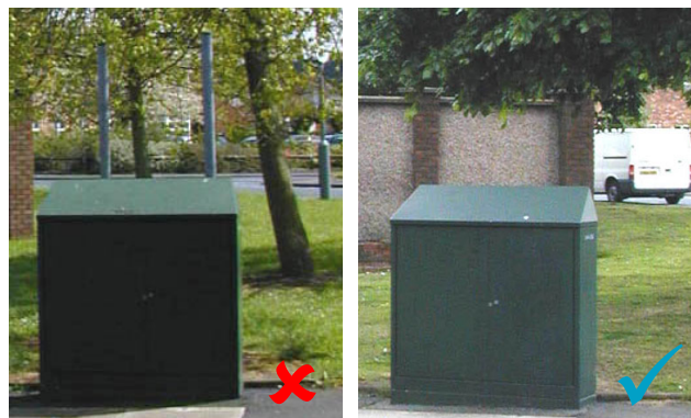
Fig 135-6. Left, defunct posts behind cabinet, subject to repeated weed-spray and conflict with grass cutter. Right, after removal.
