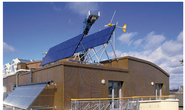
Fig 80. Temple Bar, Dublin. 'Green Building' with rooftop wind turbines and photo-voltaic panels.
