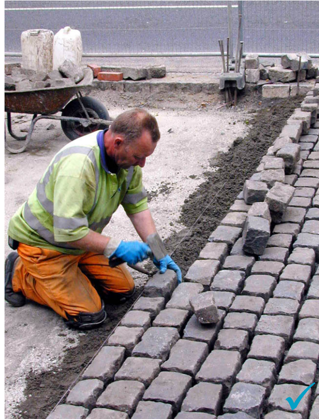
Fig.118. Relaying of setts in Westgate. Durable materials in sympathy to their surroundings.
