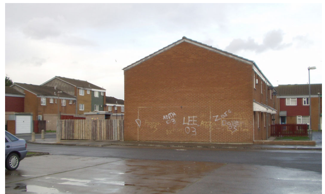
Fig 63. This blank gable, facing a turning head, invites use as a goal-mouth. A boundary adjustment would remedy this problem.
