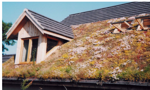
Fig 78. Detail of figure 75, showing sedum covered roof in flower. Habitat, insulation and slowing of rain run-off benefits accrue.
